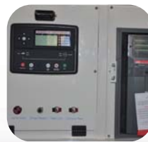
Control Panel & MCB
